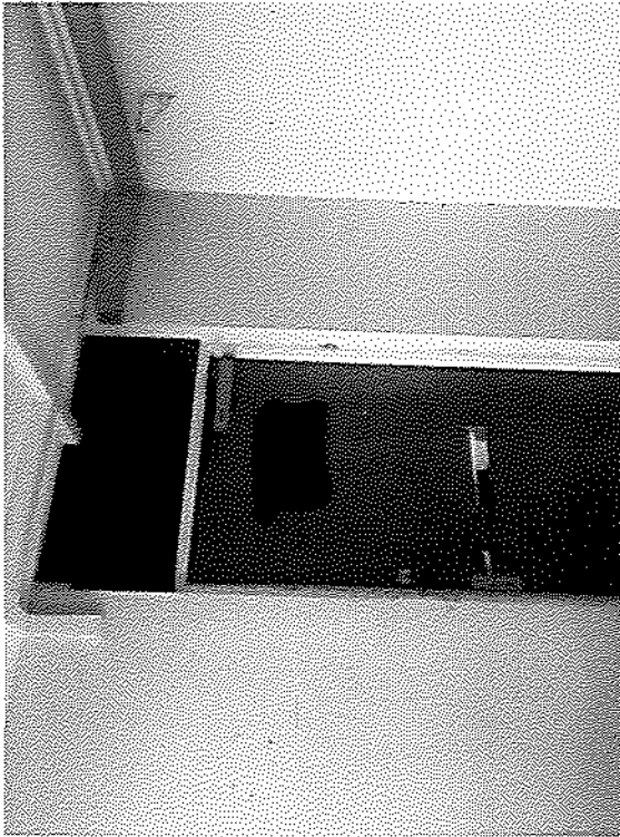
Photograph 1 – Example of a flat front door set not achieving 30 minutes fire resistance (FD30S).
