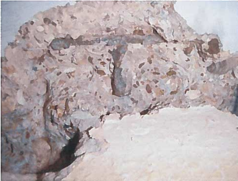
Photograph 23 Breakout U4 at wall – soffit joint at 16th floor Slab main reinforcement
