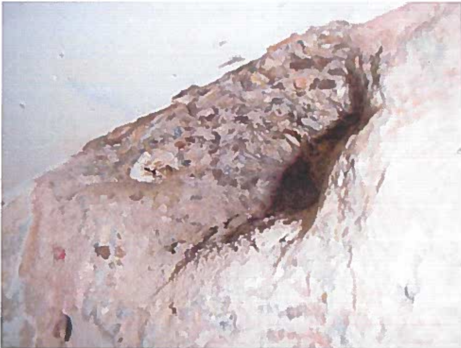
Photograph 17 Breakout U1 Ceiling level breakout showing the different concrete elements (shades) within the joint
