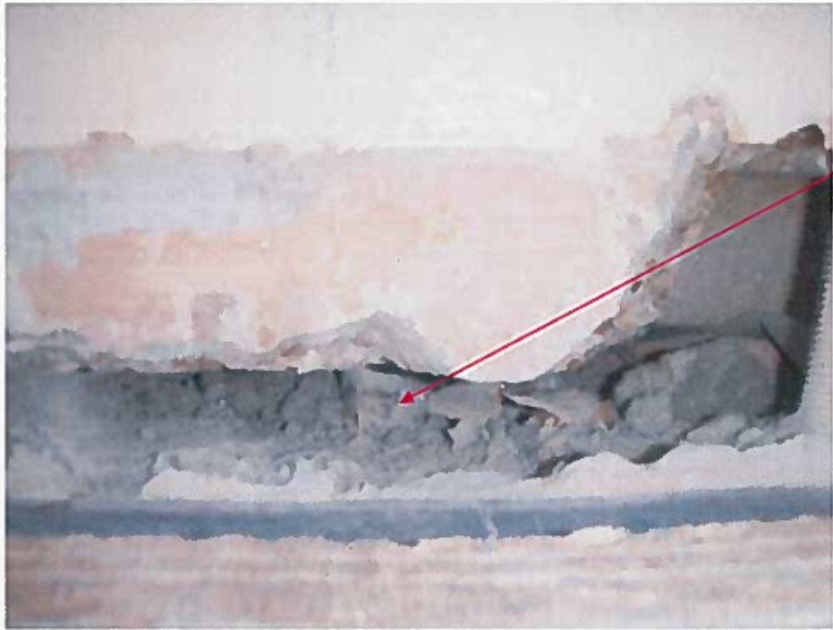
Photograph 7 Breakout L5 Exposed dowel bar
